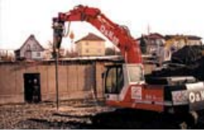
i Project Residential Building Complex Unterrohr, Kremsmünster, Austria DSI Services 2,000 m of Ø 118 mm ungrouted DYWIDAG Ductile iron piles.
