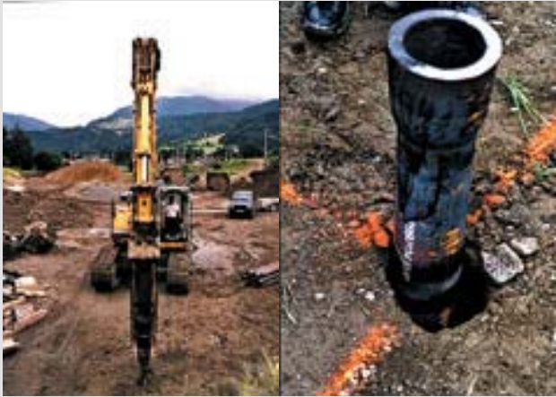
i Project Construction Site for Approval Tests, Bischofshofen, Austria DSI Services ungrouted DYWIDAG Ductile iron piles
