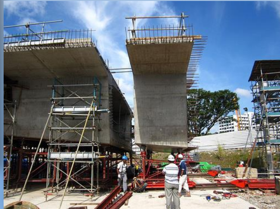
Separation of Precast Segment
