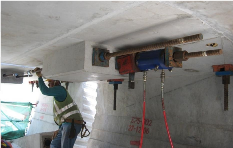
top concrete blister
