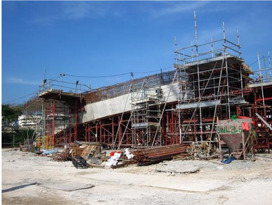
Full length precasting bed
